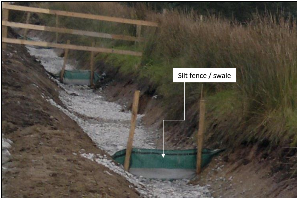
Figure 4-3 – Silt fence used in conjunction with check dams along roadside drainage channels
