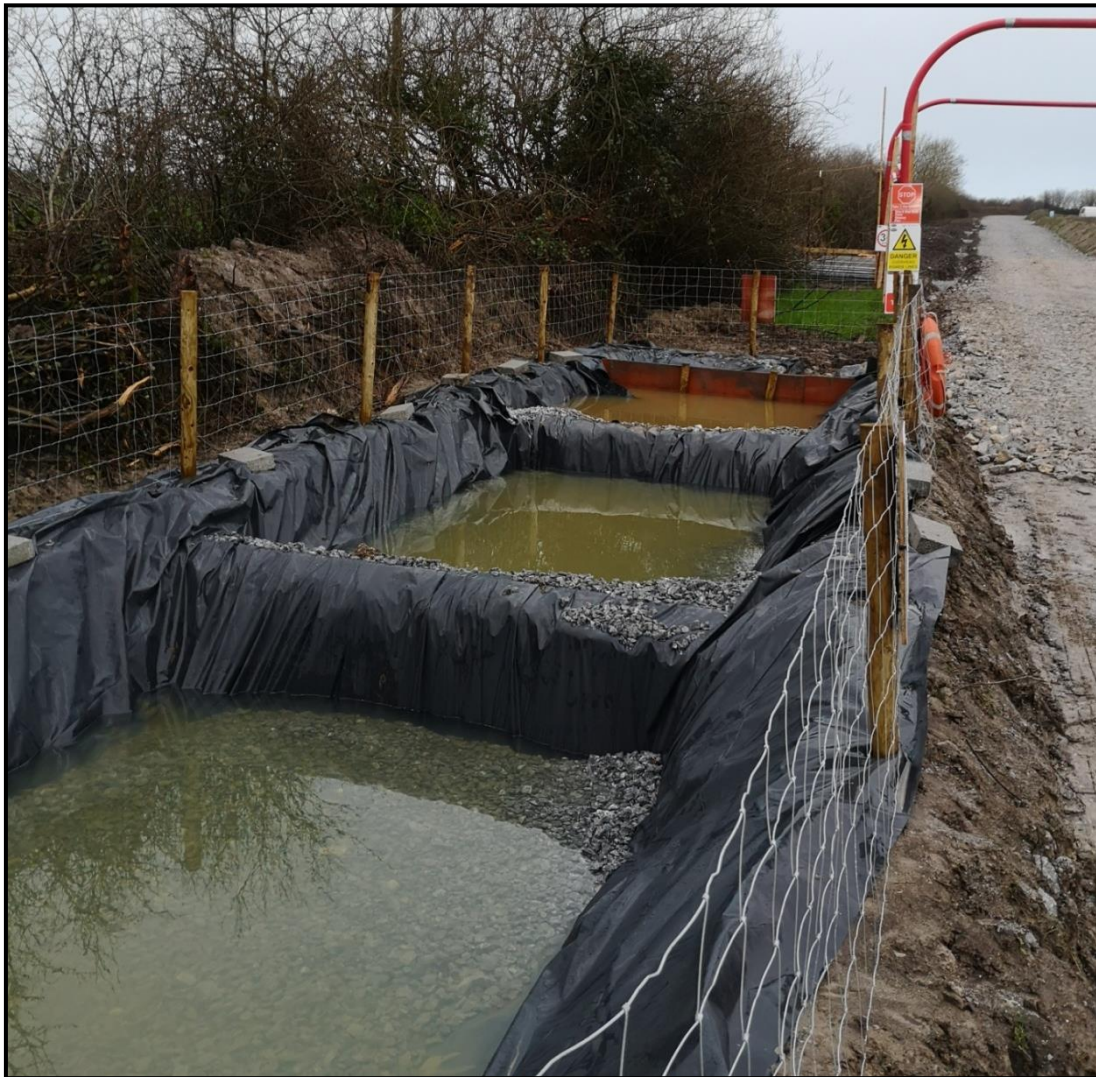
Figure 4-1 – Multi tiered settlement pond with stone filter
