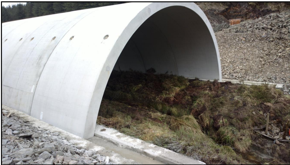
Figure 4-7 – Typical clear span pre-cast concrete units in place over an existing watercourse
